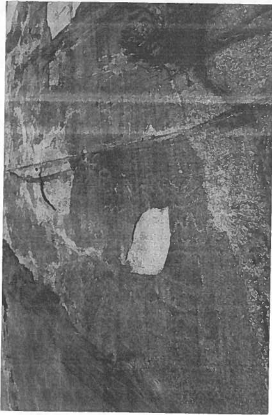
Figure 2. Natural exfoliation of rock surface has removed a portion of the Style 7 petroglyph panel at the Long Lake site, CA-PLU-4. Photo by Craig Carter, 1985.
