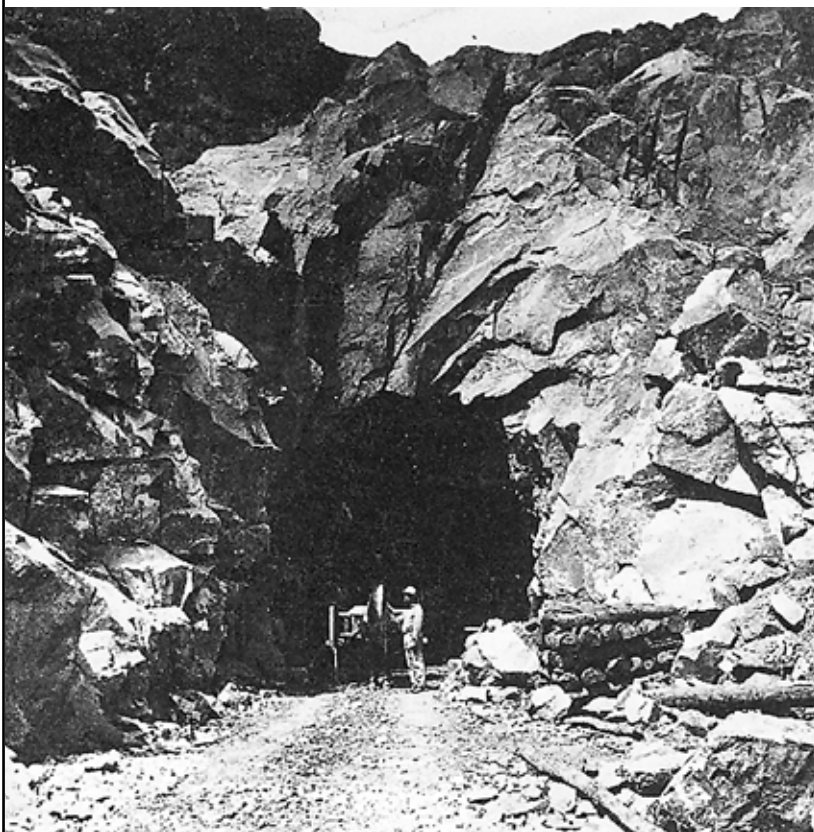
Chinese worker at Tunnel 6's east portal, Alfred A. Hart #198, CPRR photographer, portal to Tunnel 6; one half of a stereopticon slide.
