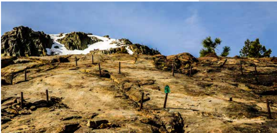
Snowshed anchors, steel rods driven into the granite, to hold the snowsheds against the lateral movement of snow outside Tunnel 6's east end below Donner Pk.
