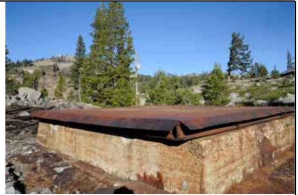
Above, the top of the the Tunnel 6 shaft. See also page three.
