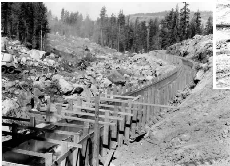
The flume diverted the Yuba River behind the Donner Summit Lodge for the building of the freeway.
