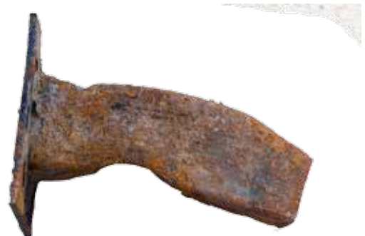
Below ruined steel cap
