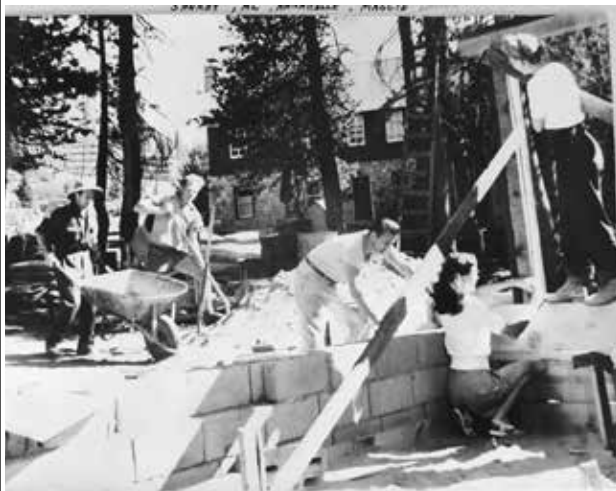
Construction work party, 1947. That's the way lodges were built in the old days.
