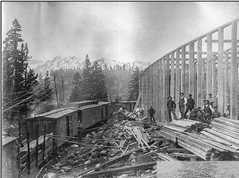
Snowshed re-construction just east of Donner Summit. Fires were the nemesis of the wooden showsheds and could take out hundreds or even thousands of feet at a time. Until the concrete sheds replaced the wooden ones there was a constant need for rebuilding.
