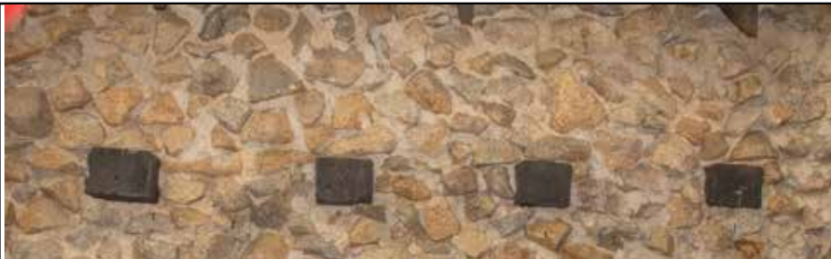
Note the differences in rock work due to different masons working on different additions to the building over time.
