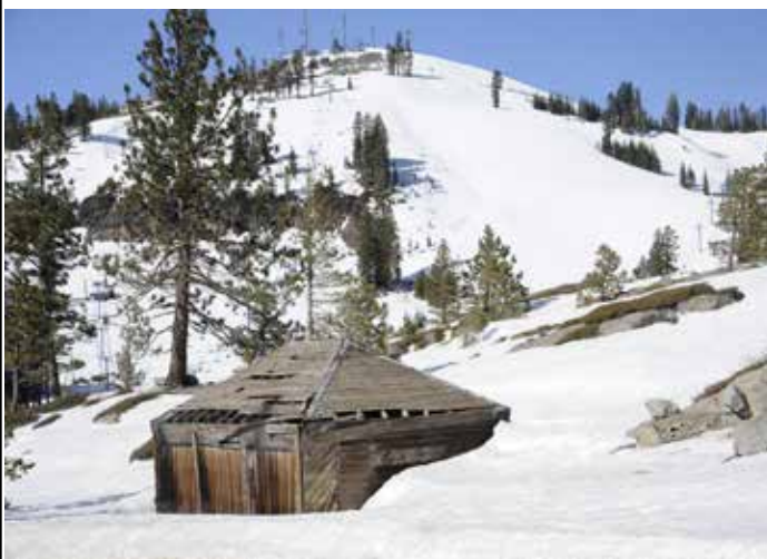
Left, the garage on Highway 40 below the weather station for the automobiles belonging to the weather station personnel. It completely collapsed in 2022.
